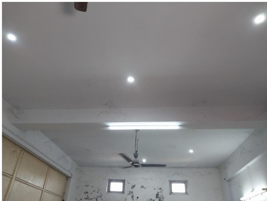
LED lights in Classrooms
